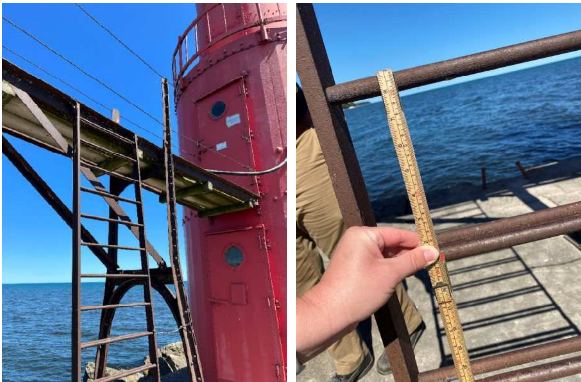
Photo 5/6 – Limited / No Access to Catwalk from Ladder; Ladder Rungs are Not Code Compliant
