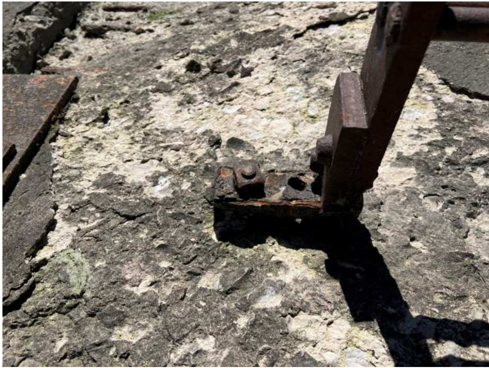
Photo 4 – Advanced Corrosion and Significant Deterioration of Critical Members Consistent Along Structure Length
