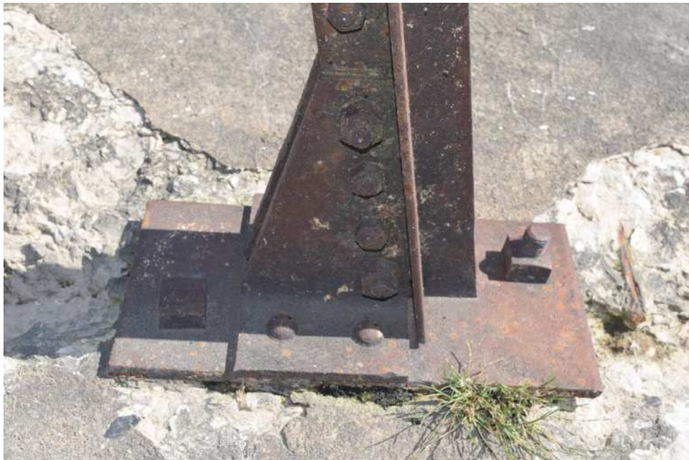
Photo 2 – Compromised Anchorage to Breakwater
