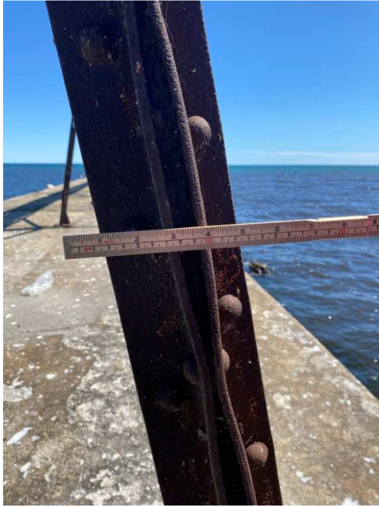
Photo 3 – Rust Jacking of Lacing Resulting in Plastic Deformation of Bent Members
